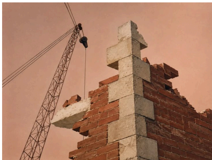
Figure 1.01b: Stones at risk of falling
